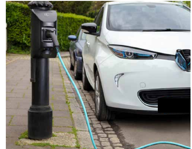
Figure 72: Example of on-street electric vehicle charging points.
