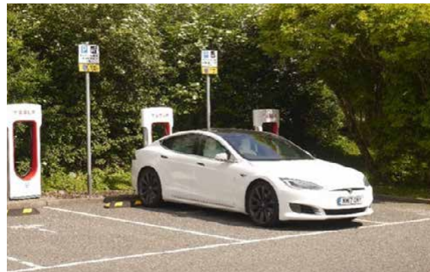
Figure 73: Example of electric vehicle charging points in a parking court.
